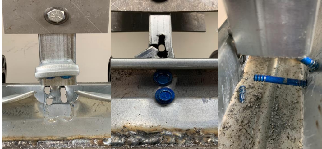
Figure 65: Similar Member Failure Types
