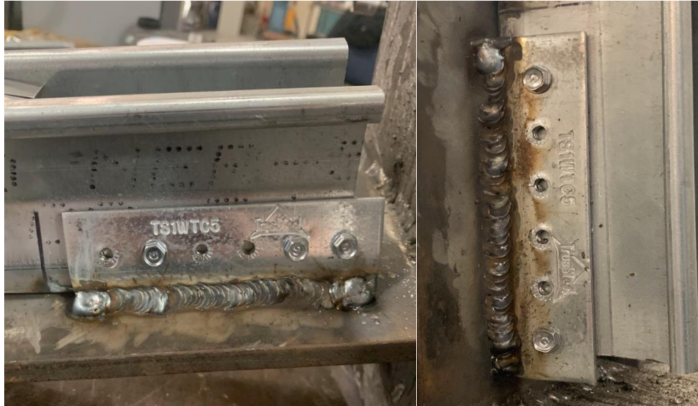
Figure 74: TrusSteel End Bearing Failure
