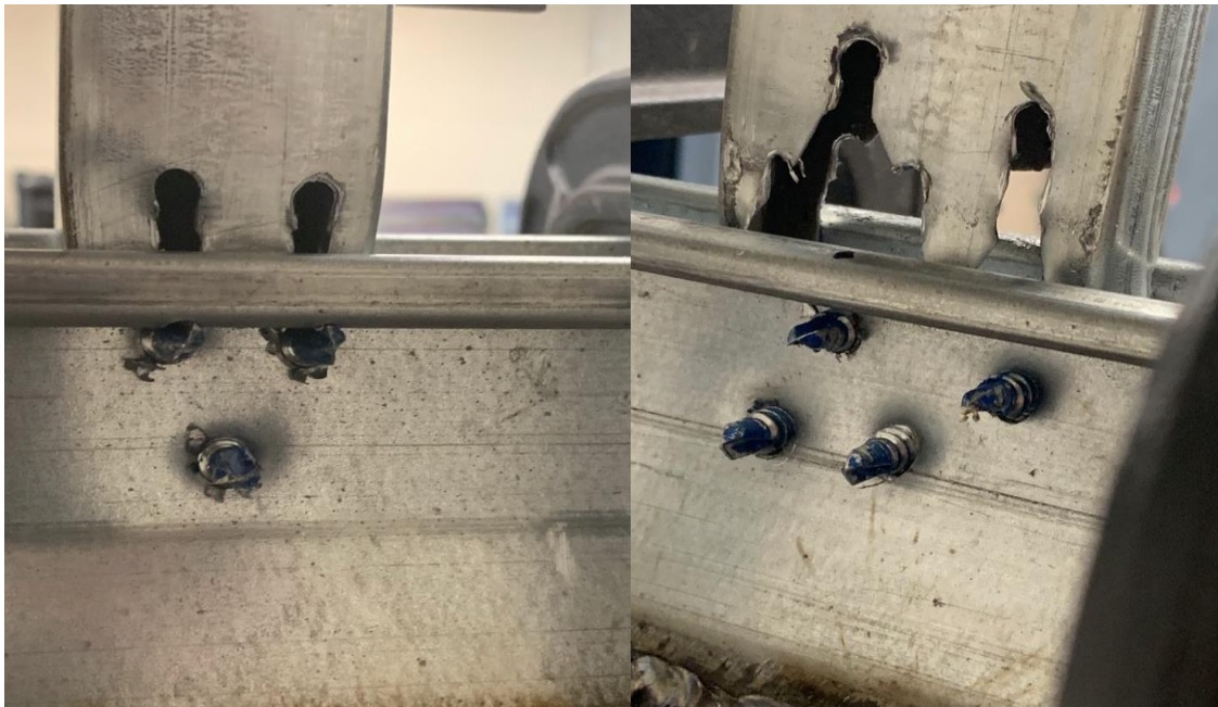
Figure 61: Bearing, Tearing & Partial Block Shear Failures
