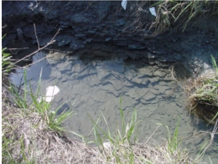
Figure 26 – Exposed area showing shale that is underlying highway in District 4.
