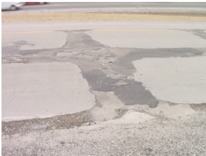
Figure 27 – Heave in I-435 due to underlying expansive shales.
