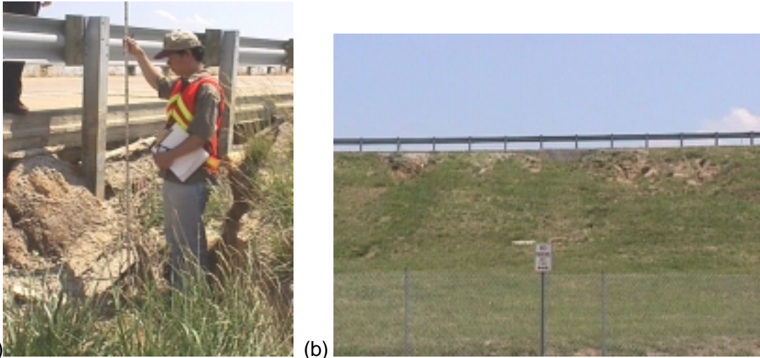
Figure 15 – (a) Erosion at the edge of shoulder concrete on Spencer road ramp on to Mo-370. (b) Erosion problem near I-170 and I-70 intersection.
