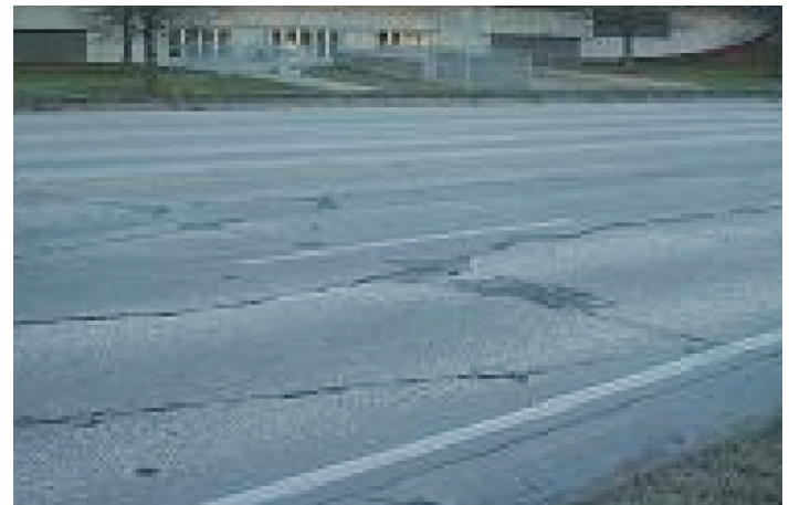
Figure 4 Pavement Problems Observed During Survey
