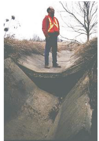
Figure 3 Erosion Observed During Survey
